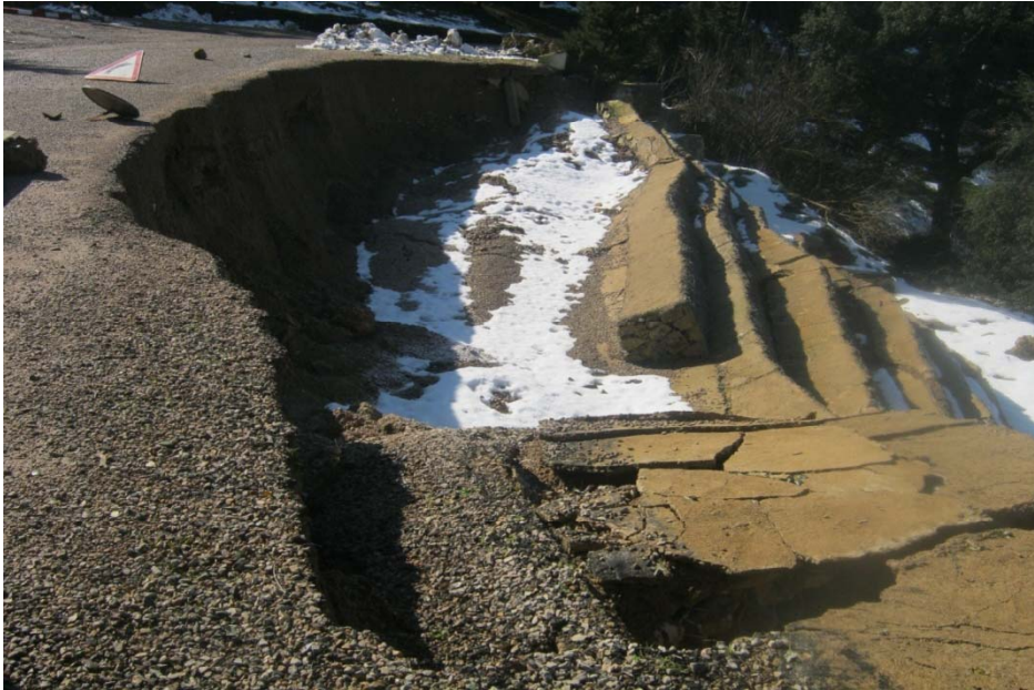
Photo 1: Reactivated old landslide
