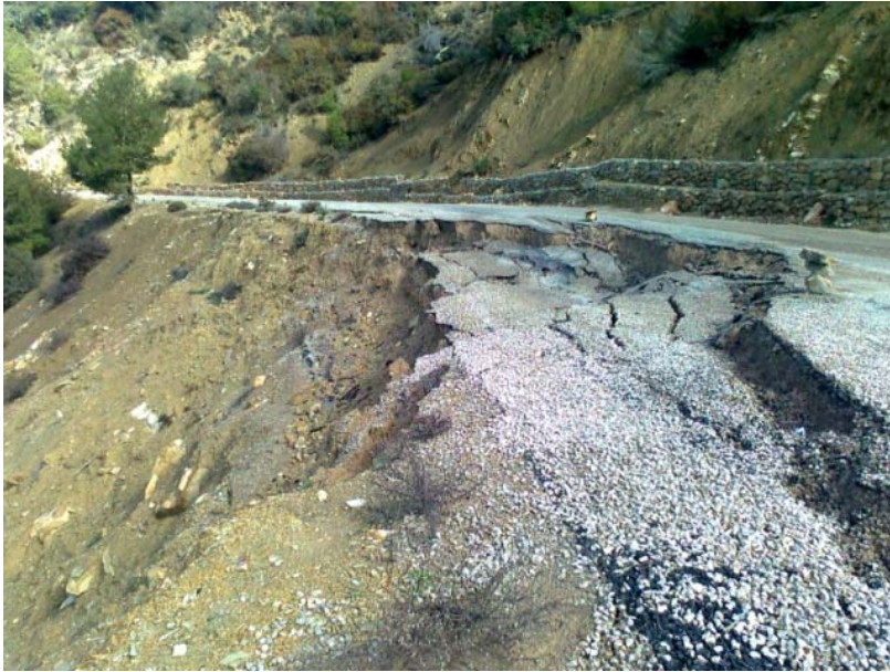
Photo 3: Landslide: occurred failure
