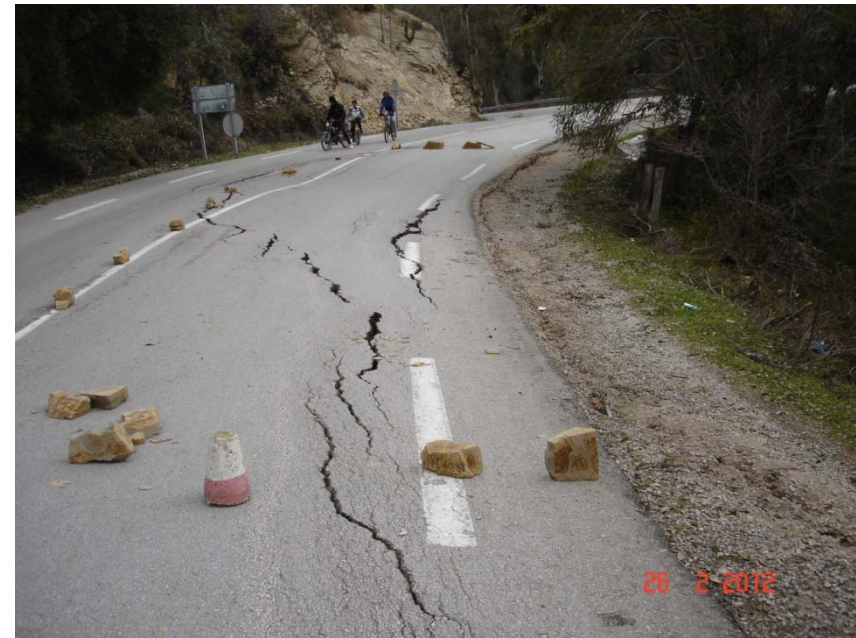
Photo 2: Landslide: prefailure state
